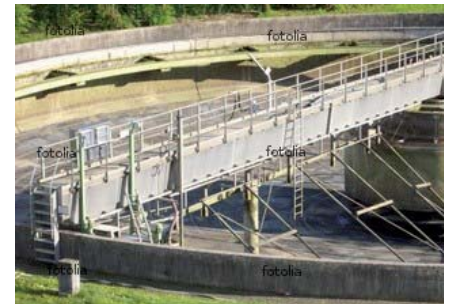
Sewage tank with scraper
